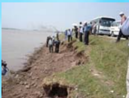
The 650m of central seadyke in Thai Do Commune- Thai Thuy District - Thai Binh Province eroded due to Storm Damrey as a result of mangrove absence (Photo: Phan Hong Anh taken on 10/10/2005)
