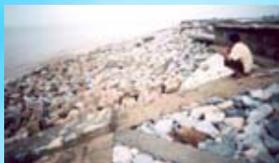
Sea dyke broken at Cat Hai where there were no mangroves
